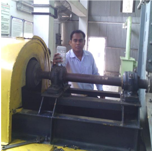
Bearing Vibration Measurement
